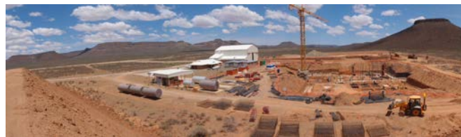
Figure 2. The mid-phases of the Karoo Array Processor Building (KAPB) construction showing soil berm from earth excavation, some connected reinforcing, the ground level with earth mat and bond-ring conductor.
